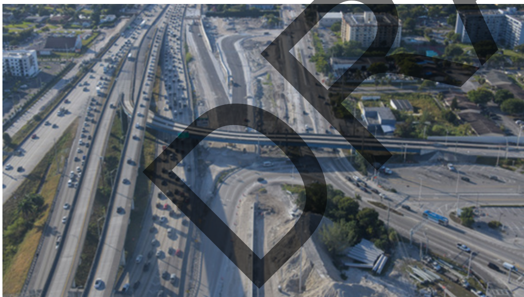
Construction of "Ramp O" Southbound off-ramp from I-95 to US-441 / NW 7th Ave
